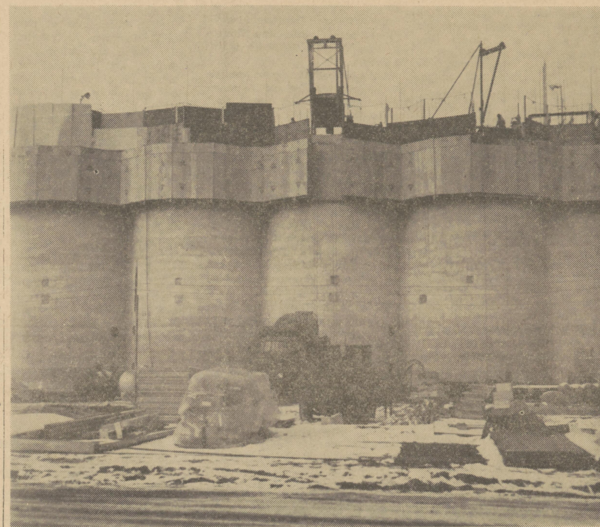
GETTING UP IN THE WORLD — Construction of the 400,000-bushel grain elevators of the Kilen Grain Company as of last Friday. Pouring of concrete for the 111-foot high towers was ended Monday night. However, pouring of concrete for the tops was scheduled to begin Wednesday. Installation of machinery will be completed by May. Borton, Inc., of Hutchinson, Kan., is the contractor.
