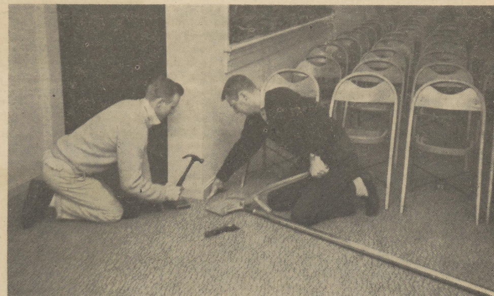
Putting finishing touches of carpet in the Main Chapel at the J. Millard Cooper Funeral Home
