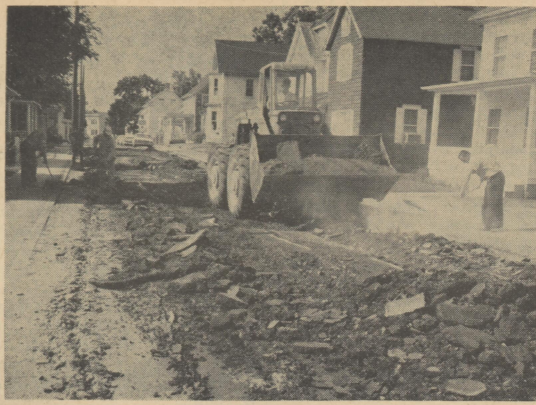
DIPSIDOODLE — At intersection of Liberty Street and Fleming Street and Weiner Avenue will be eliminated for h-with. A construction company has started going away with the dip.
