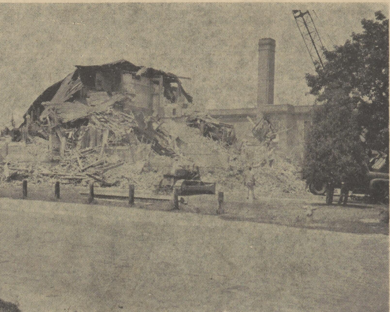
1912 SCHOOL RAZED—Work underway as part of program for new high school, practically completed.
