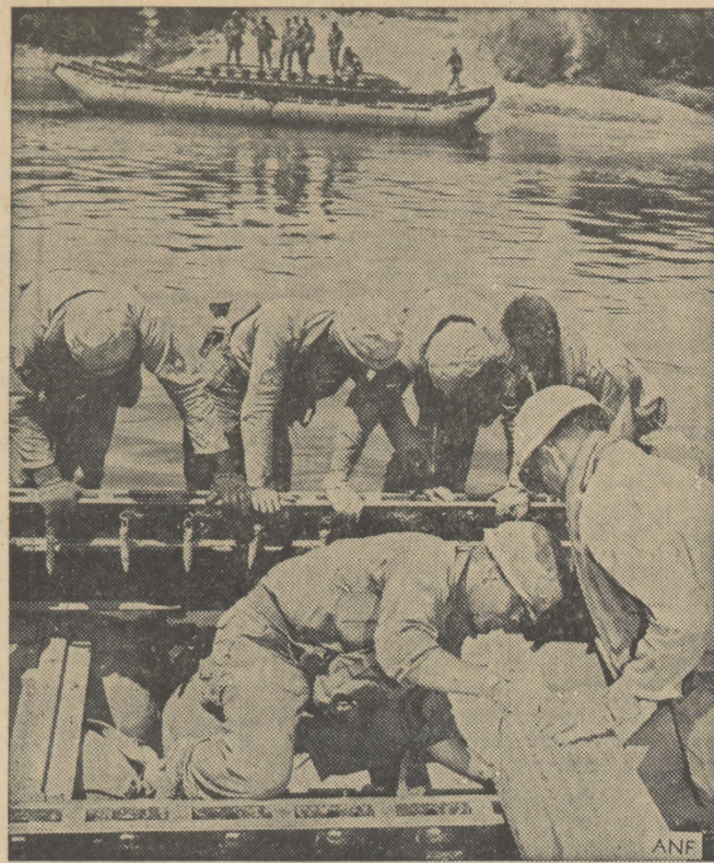
THEY SHALL PASS—Engineers from the 17th Engineer Battalion, Fort Hood, Texas, assemble a pontoon bridge to be used by the 2d Armored Division in crossing the river into the heart of the enemy country Calonia. The bridge will support the M-60 Main Battle Tank, which weighs 52 tons.
