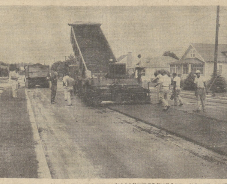
WORKMEN OF SEAFORD CONSTRUCTION COMPANY Seaford, laying a 3 1/2" "hot-mix" asphalt road bed on Delaware Avenue, from curb to curb. Center Street will receive the same improvement under the $132,000.00 construction project awarded by The State Highway Dept. Price photo
