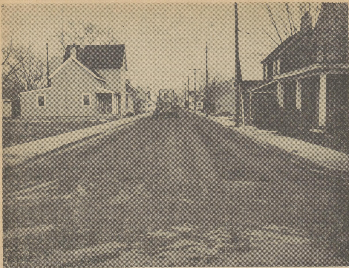
THE NEW LOOK — Goes on Wolcott Street on curbing, blacktopping. A final coat will be applied in the spring after the roadbed has settled. In the meantime, sidewalks are being installed. Price photo
