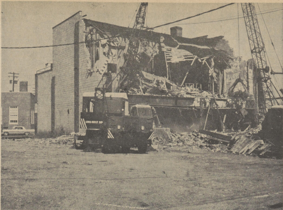
WHAT GOES UP MUST COME DOWN—The Reese Theatre is being razed to provide a parking lot for Peoples Bank. This is a rear view of the building. Price photo
