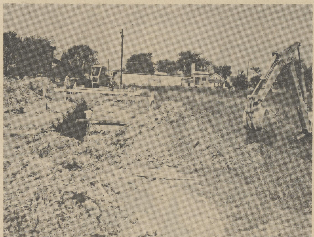
GETTING TO THE BOTTOM OF THE MATTER—The community's sanitary-sewer improvement program was well under way this week with a trench being dug on Reed Street from South (Peck Ave.) St., to Clark Street.
