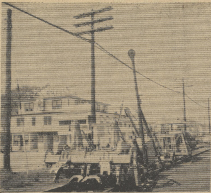
WHAT ARE THEY? — They resemble a pile of trash but there are three vehicles here which aid the track crews of the Penn Central. The front vehicle extracts railroad ties; the middle vehicle, hardly discernible here, moves ties, and the last vehicle tamps spikes into ties. Journal photo
