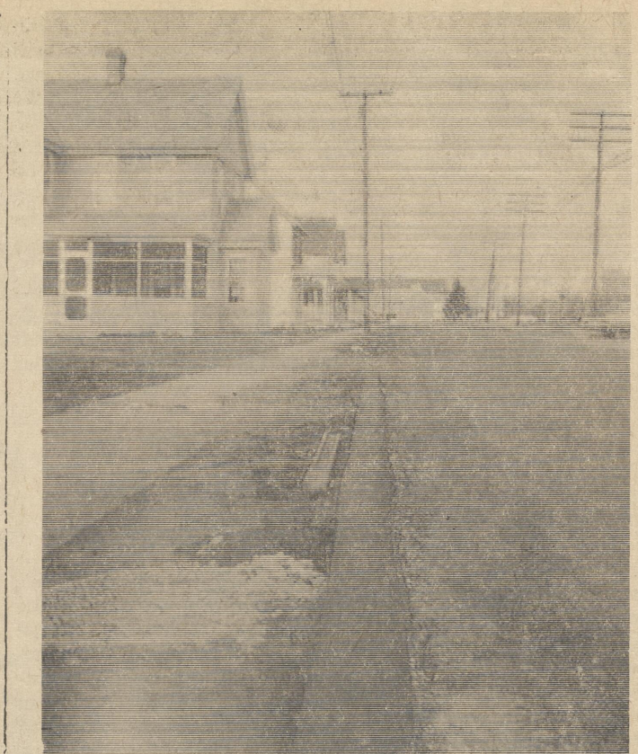
THE RIGHT TRACK? —If it proves lasting, this black-top curb will be economical for the City of Harrington. It will cost less than concrete curb and can be laid quickly. This curb is on Railroad Avenue.
