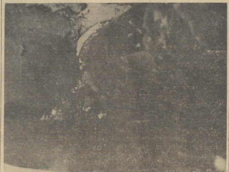
DEFECTIVE FLUES CAUSE FIRES—This photo, by Fire Chief Robert A. Wilson, shows entrance of a stovepipe at a defective flue, cause of a fire at the home of Kathryn Wynn here Christmas Eve.
