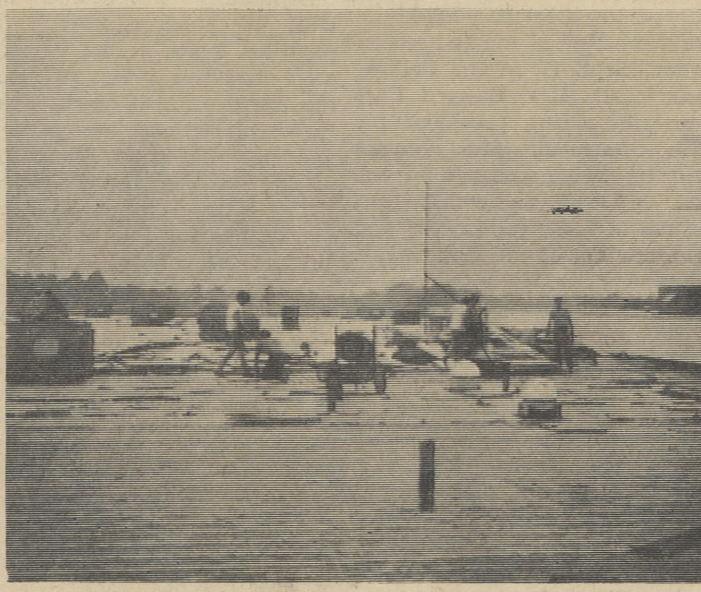
A NEW ROOF AT LAST—Workmen of the Tri-State Roofing Company of Seaford began tearing off the old roof and installing an entire new one at Lake Forest High School. The contractor says that the roof can be installed in 35 working days.—Price photo.
