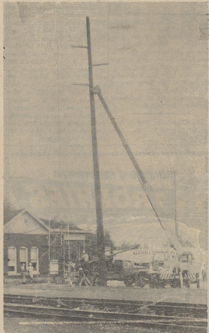
One of the many electric poles being erected for Delmarva Power by C. W. Wright, general contractors, to feed the new substation for Harrington located below Harrington on Farmington road. The new line is coming from the Cheswold Substation and will be along the railroad right-of-way line. The line is not connected with the railroad. It will carry 138,000 volts and will be a major tie for all of Delmarva's plants from Wilmington to Millsboro to Vienna, Md.
