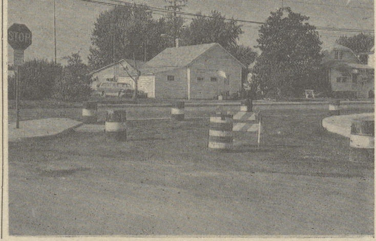
The New Reese Avenue intersection. Photo shows what it will look like to turn off Reese Avenue (going west) onto Commerce St.
