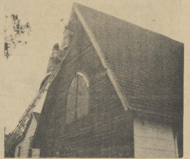
Kenneth (Snooky) Collins of Harrington Fire Co. with axe as top man on the ladder looks for the source of the fire to the former home of St. Stephen's Church on Fleming St. in Harrington. The fire was confined in the roof area of the building.
