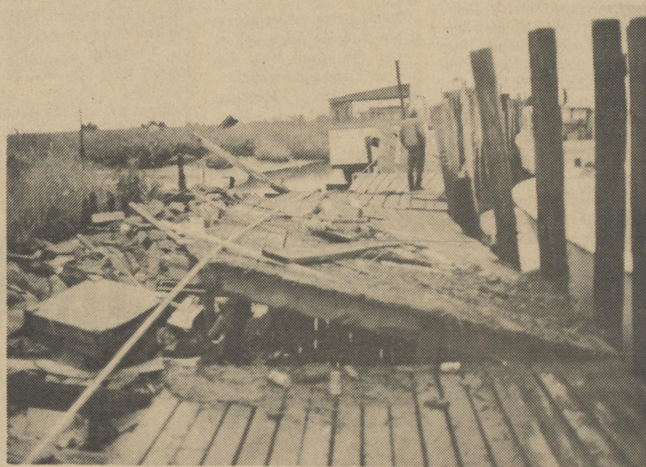
Some of the damage to the dock and wharf at Mispillion Lighthouse. This scene was repeated along the coastline.
