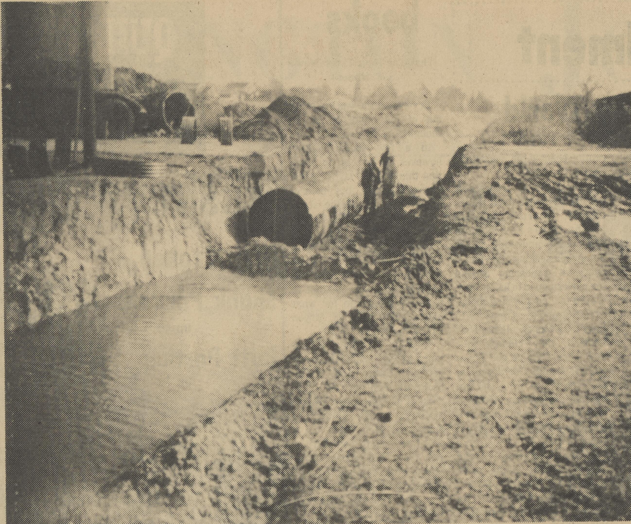
Work continues on the Browns Tax Ditch. This scene is near Second Avenue in town.
