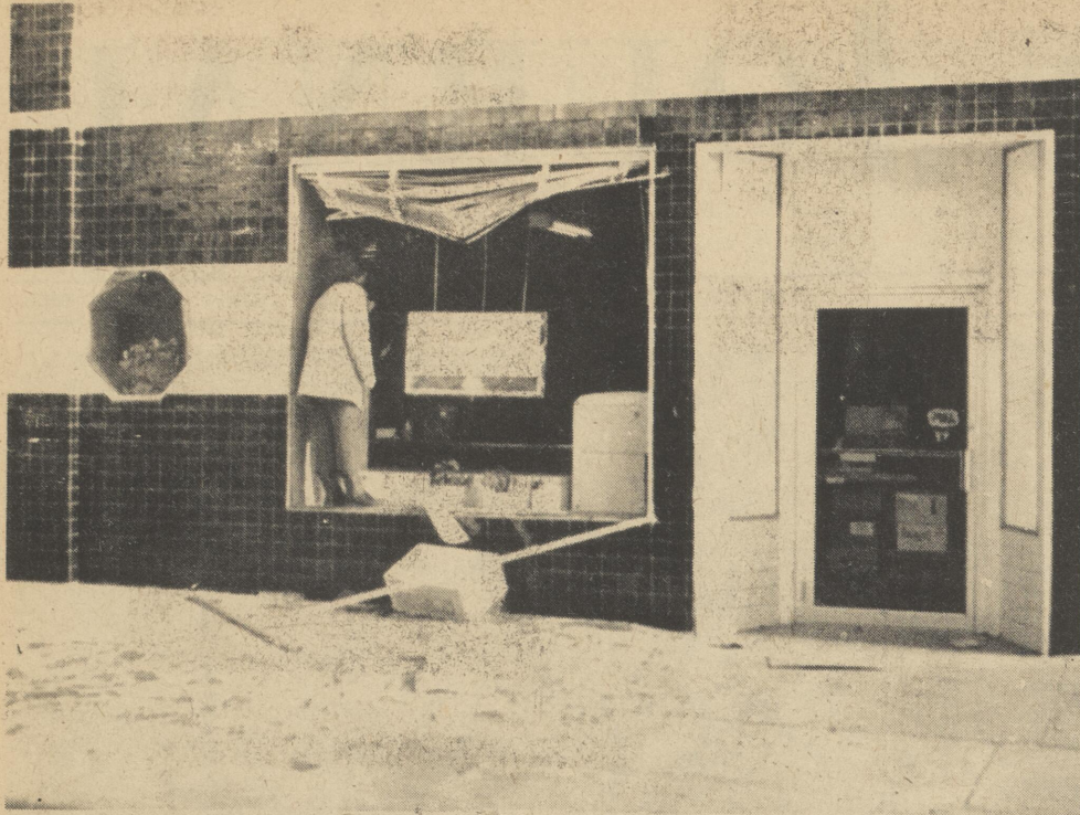
This is the scene of the Pensupreme Friday morning, following the breaking of the front window. The break was caused by the high winds that struck the area.
