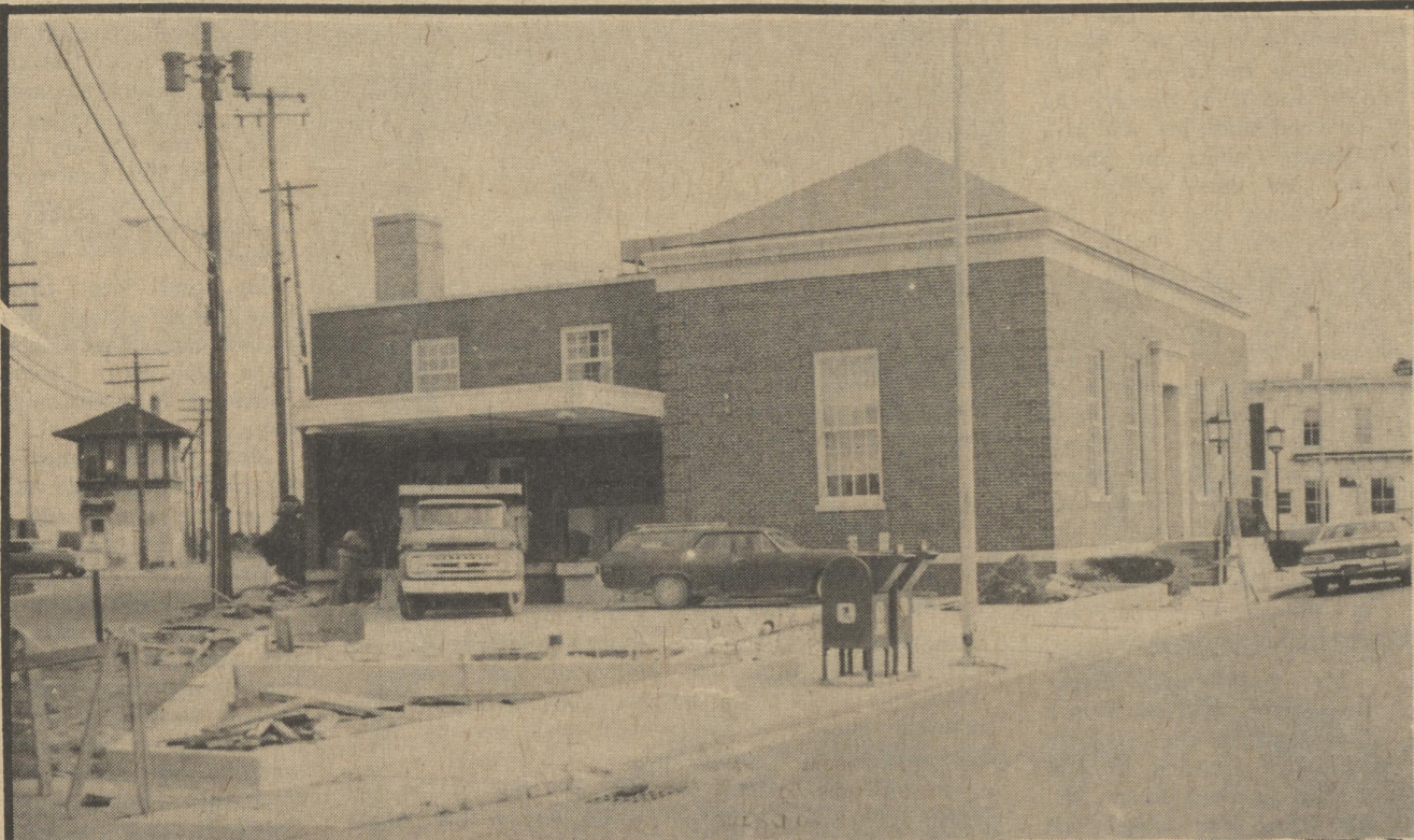
Work continues at the U.S. Post Office in Harrington. A new flag pole is scheduled to be placed on the Clark Street side of the building and the parking
