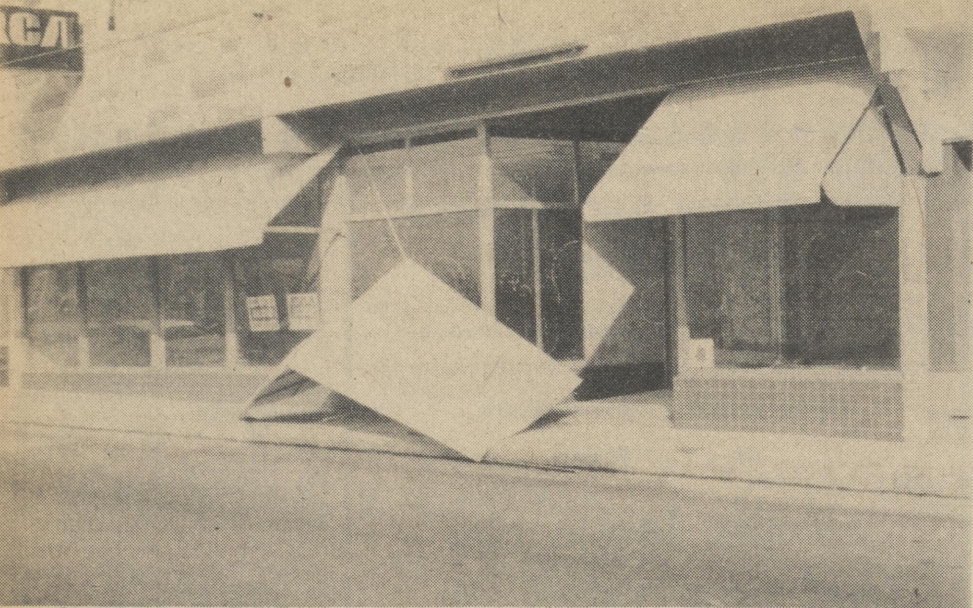
The Shaw Furniture Store building shows some of the damage caused by last Thursday's thunder storm. There were reports of other minor damages and power failures.
