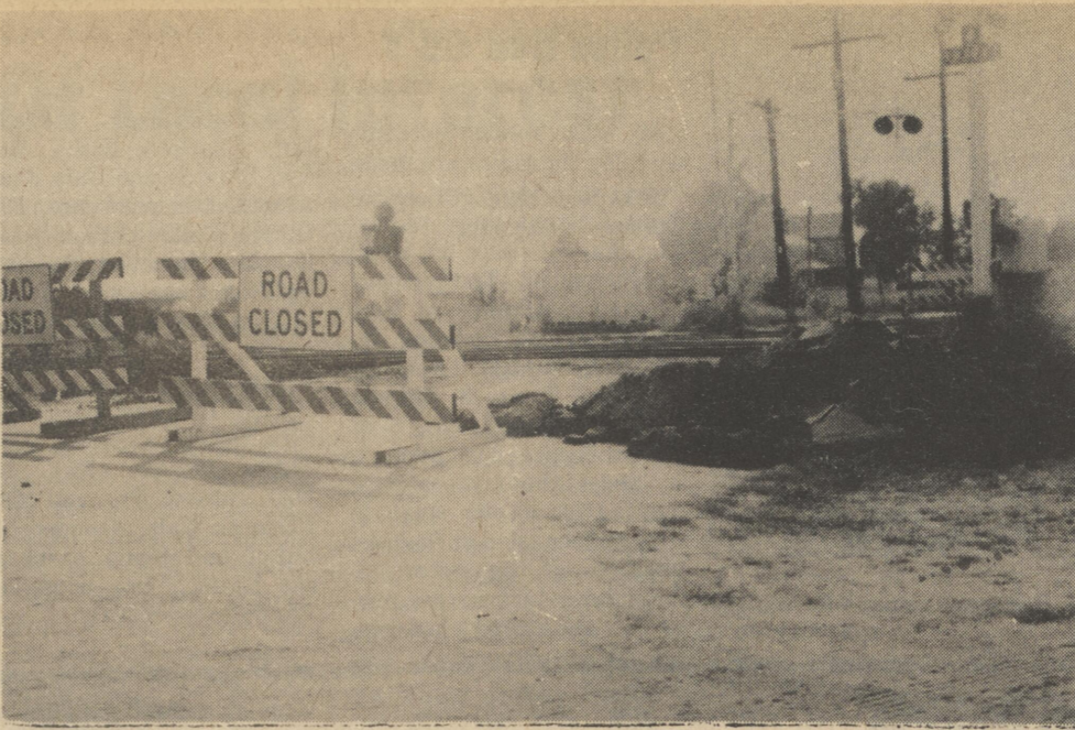
Fairground Road is closed during work on the crossing there. It will cause inconvenience to race track users next week, among others, as a detour is necessary now.
