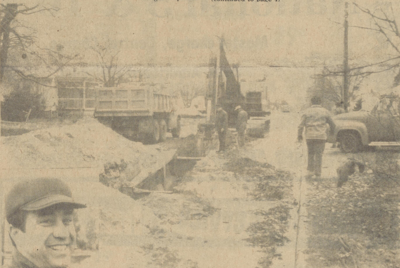
Work began last Thursday in Frederica on the installation of the sewer system for the Town. The construction is being carried on by Central Construction Company of Hazlet, N.J. The owner of the company is Arthur Carpinello whose picture appears as an overlay in picture. Carpinello has been working at this trade for 20 years. This is the futherest south which they have
