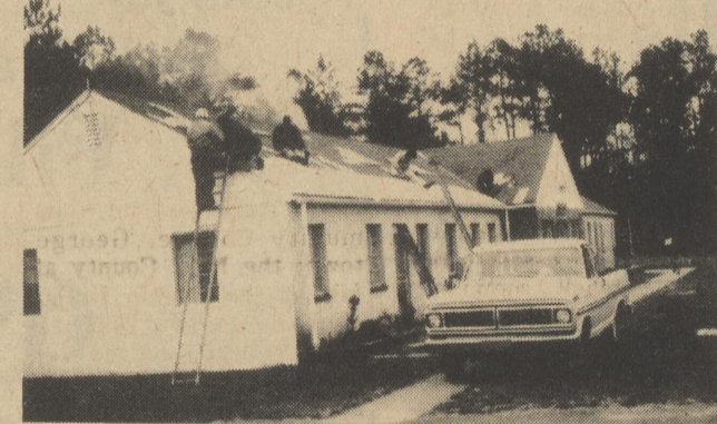
Volunteer workers, participating in a project started by District 22 Lions Clubs of Delaware, rattle the roof of the Arts and Crafts Building at Camp Barnes. After a lost election, the project was taken by the Rehoboth Beach Lions Club, but it is their hope that the other Lions Clubs in the state will continue to support the endeavor.
