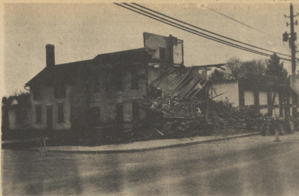
This old property which is known as the Luff property in the town of Felton, has needed some upgrading for years. It has recently been purchased by the Felton Fire Co. and was demolished last week the behest of the new owners.
