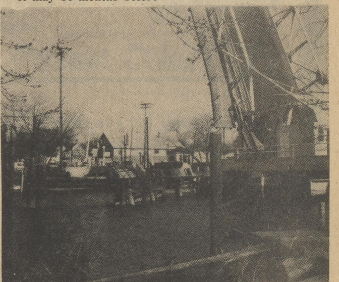
Yes, the bridge is up but don't wait - unless you plan to camp for quite a while. The span of the bridge at Denton stands drawn, revealing its west end which crumbled into the Choptank Monday. Since there is no word on when repairs can be made, extensive detours will be necessary for those traveling into or through Denton for an indefinite period.
