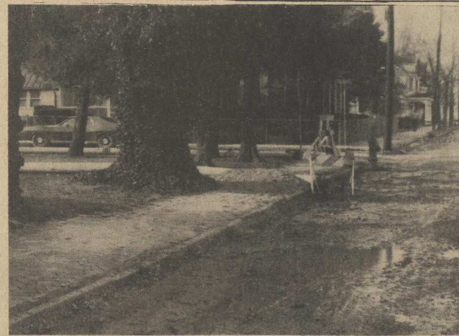
The Frederica sewer installation project continues, with some inconvenience and torn up streets at the same time. The project nears completion, however, and the signs of utility construction as viewed on Market Street will be only a memory when the job is done.
