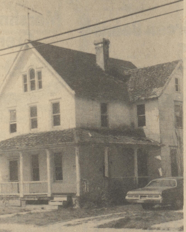
This property of Commerce Street, another van Geisel property will also face demolition sometime this month.
