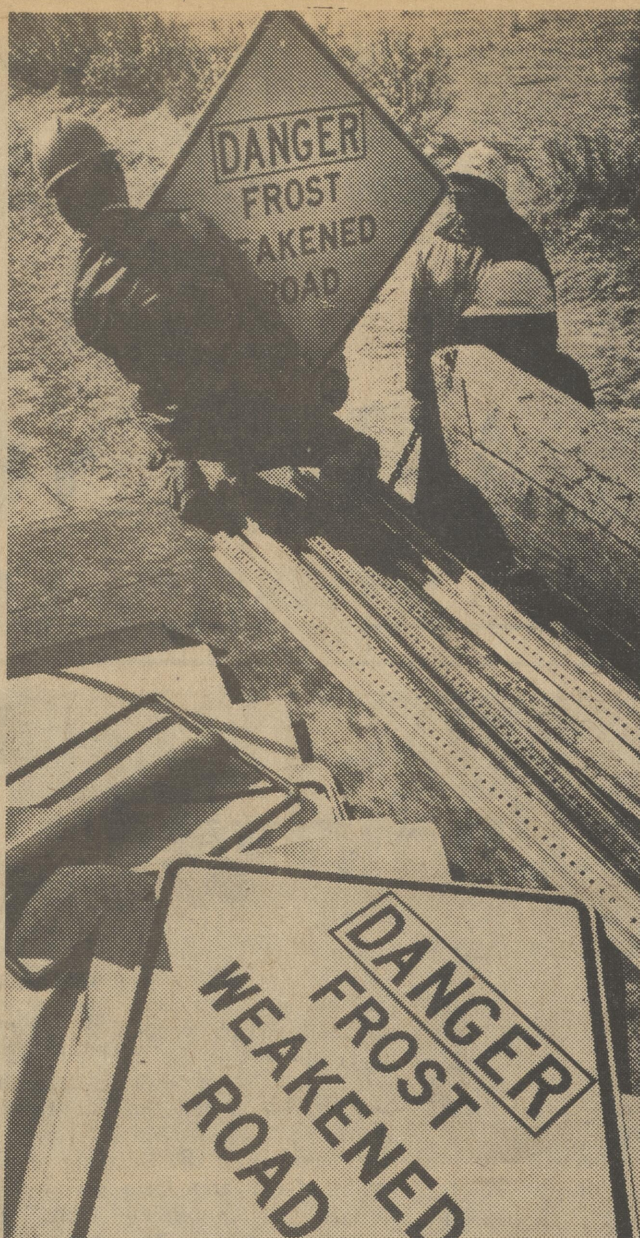
Division of Highways Maintenance crews are shown erecting the Department of Transportation's newest traffic sign warning of rough road conditions ahead.
