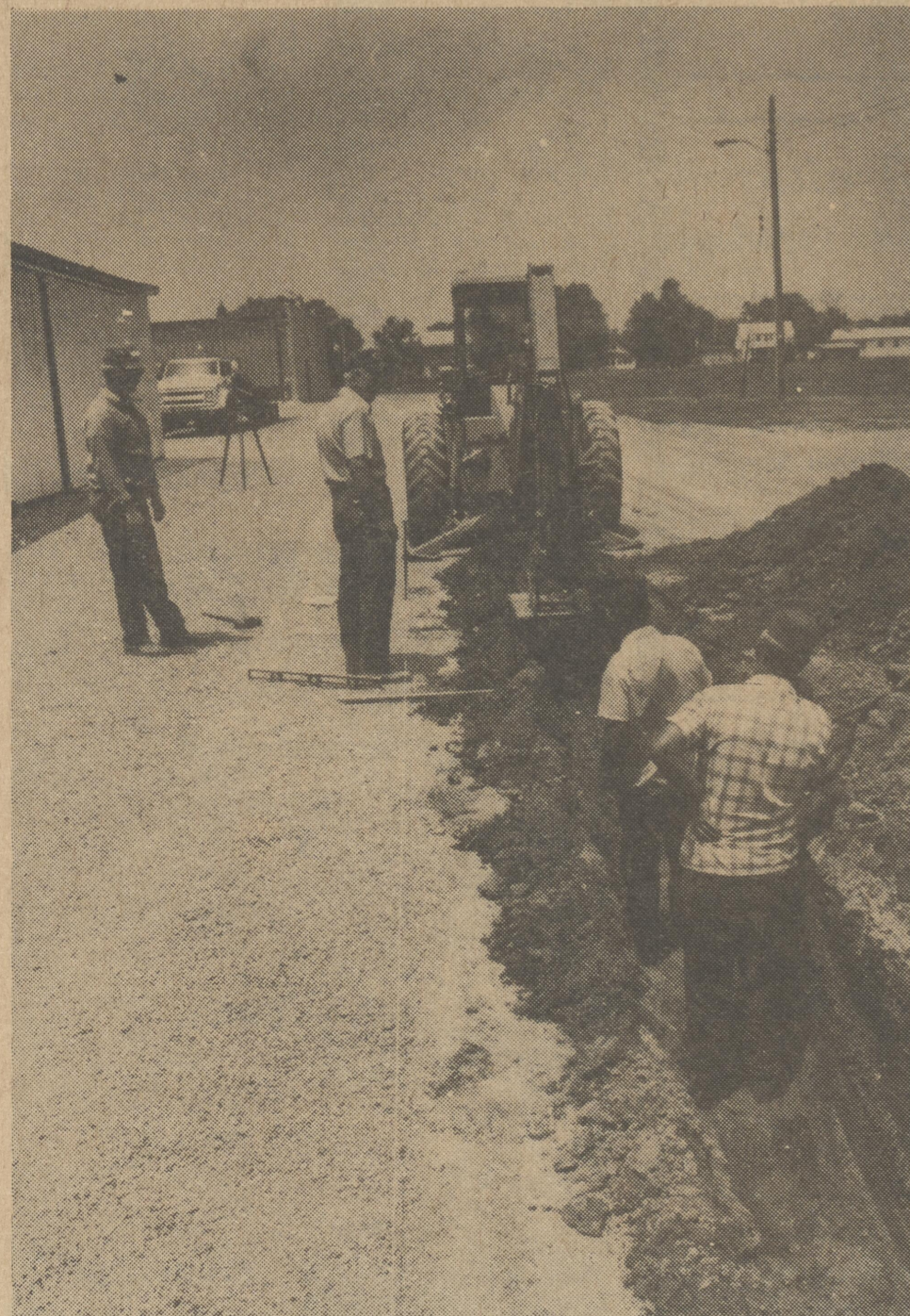
The City of Harrington has begun installing a new sewer line which will eventually hook up to Walter Messick's antique museum. The new line will also have the capability of additional hookups in case of any additional building in the area. Above, the city workers have completed about half of the digging for the 300 foot section. (Staff Photo by Ray Blanchette)
