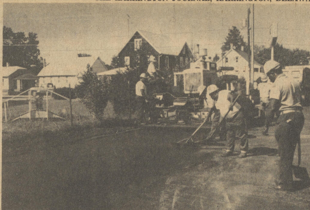
Saying this is another improvement for the city, Earl Quillen had the parking area paved in front of his Dairy Market Store on Dorman Street last week. The work was done by George Lynch of Dover.
