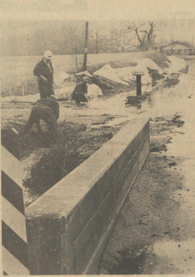
Members of the State Highway department work on a bridge on the Frederica-Harrington Road just below the ILC plant before it washes out. Working on it are Henry Queen, supervisor, standing, and Carl Legates and David Venerble. With all the rain and melting snow the bridge came very close to washing out.
