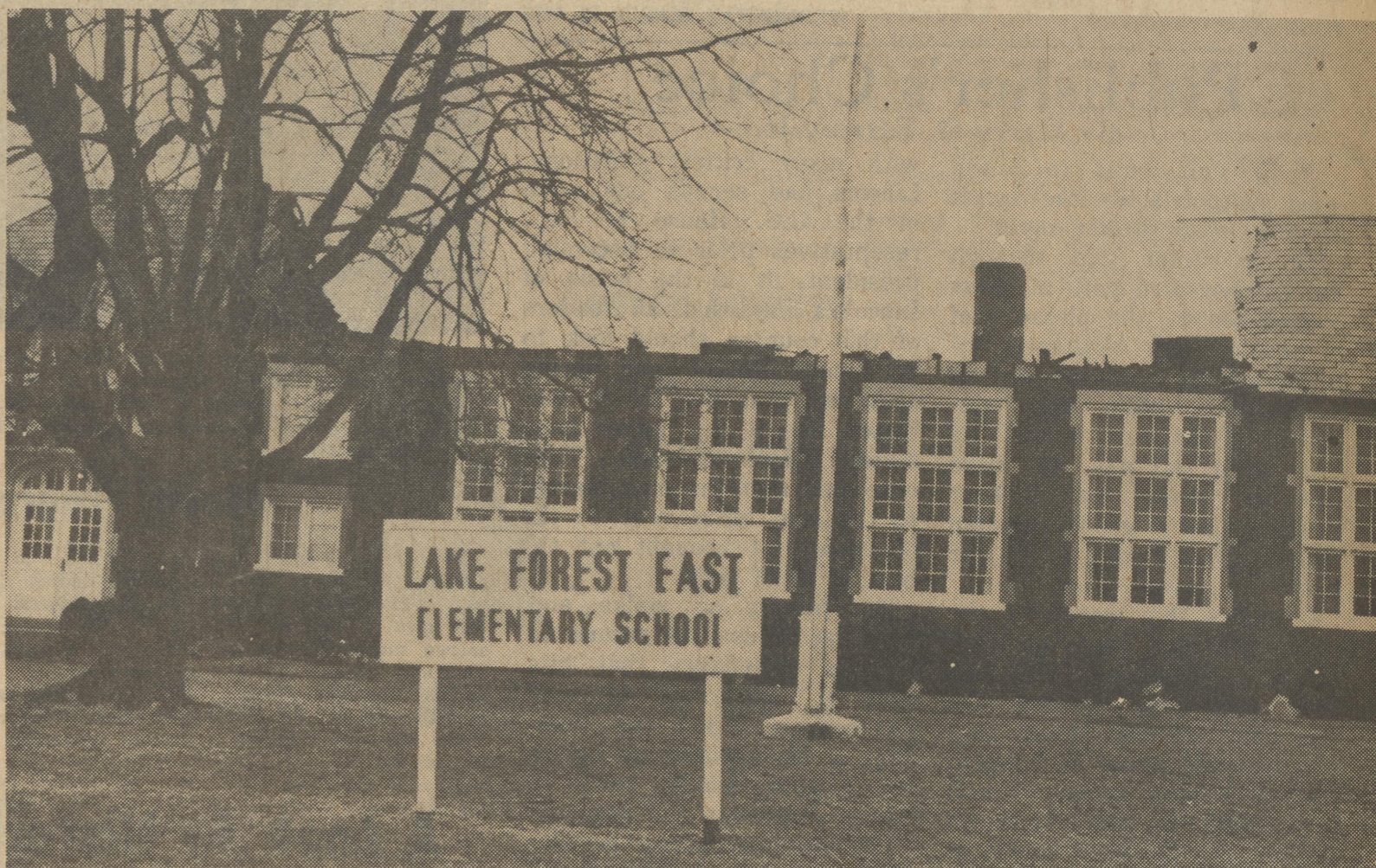
Only the Chimney remains standing in the background of the Lake Forest East Elementary School in Frederica after fire severely damaged the gymnasium area and roof on Thursday evening. Little damage was done to classrooms with most of it being just smoke and water.
