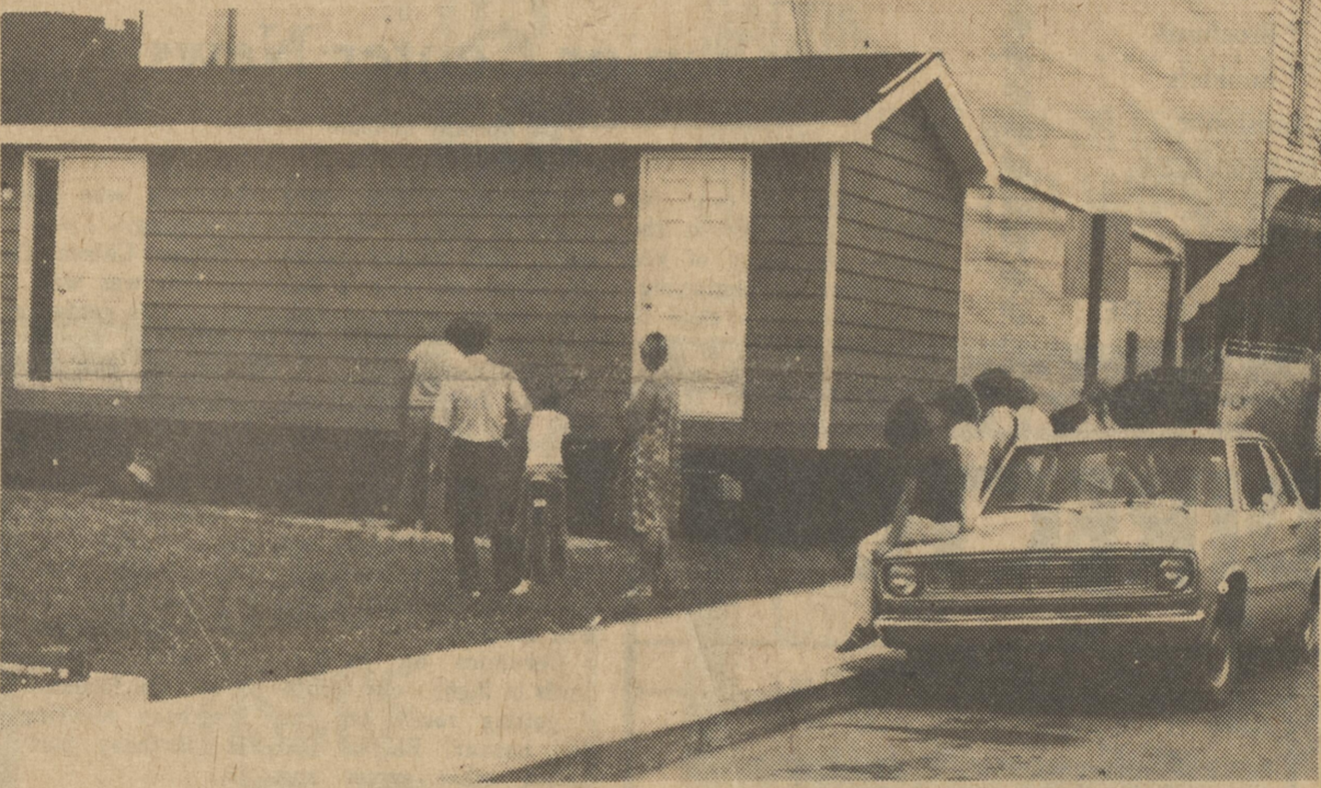
Bystanders paused to watch the arrival last Wednesday of the new modular unit for the Harrington Library. Also watching as workmen prepare to ease the unit onto its foundations are City Councilman William Shaw, and Megan Shaw, member of the Library Advisory Council [center, right].
