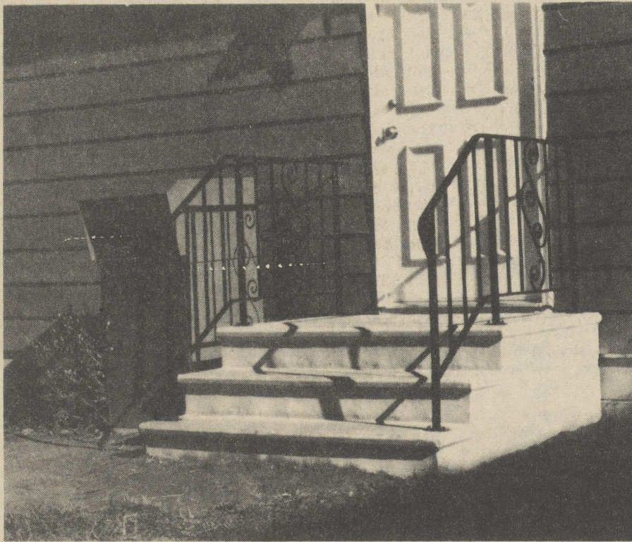
They're beautiful - New concrete steps complete with sturdy rails welcome visitors to the Harrington Public Library. The steps were moved in just this week.
