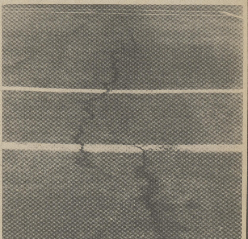
Here's a shot of a section of the tennis courts at the Chipman School. These types of cracks and depressed surface are in evidence on both of the courts.
