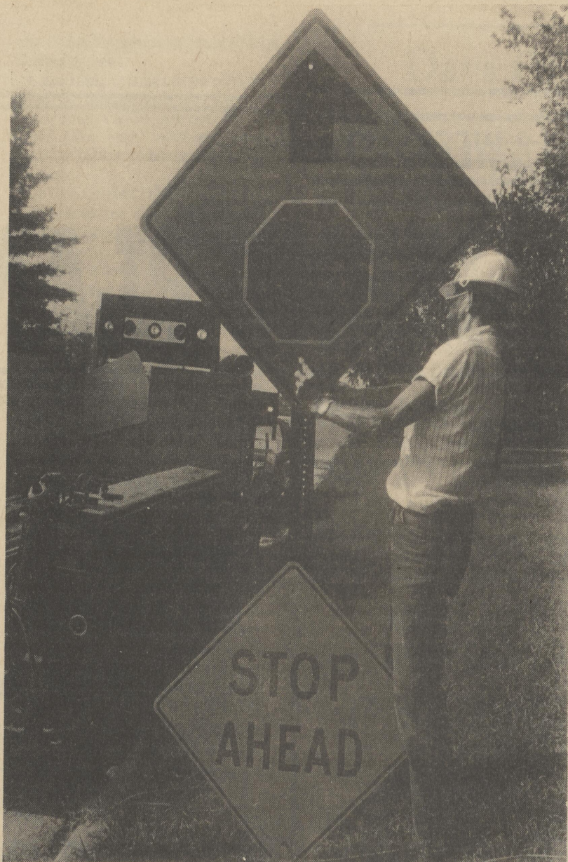
Division of Highways' crews are shown installing the new "wordless message" traffic sign indicated STOP AHEAD. Installation on a statewide basis is already underway and is part of the international movement towards uniform wordless signing.
