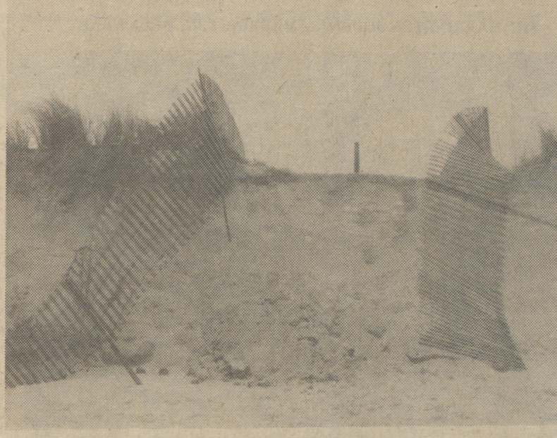
Soil erosion to the beach 1 mile north of the Indian River Inlet Bridge shows how badly the beach is eroding away. Photo by H.G.F.
