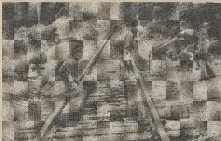
Conrail workmen led by Walter Lekites, left, bending, rebuild a railroad crossing east of Houston. Photo by HGF
