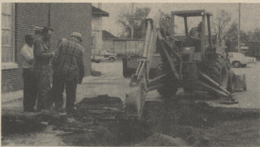
Bob Hassett operating the backhoe in the parking lot of former Peoples Bank on Monday, located the water line leak. "It was a small pin hole in an old service line," Hassett said.
