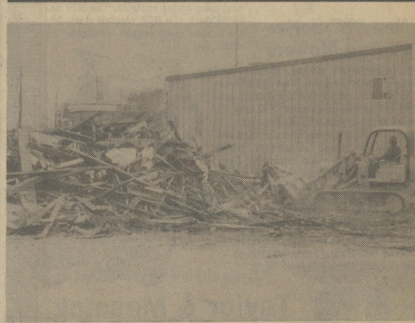
Workmen clean up the debris after demolition contractors razed former city hall on Fleming St. last week. The building was the former home and office of the late Dr. Hewitt Smith. Photo by HGF
