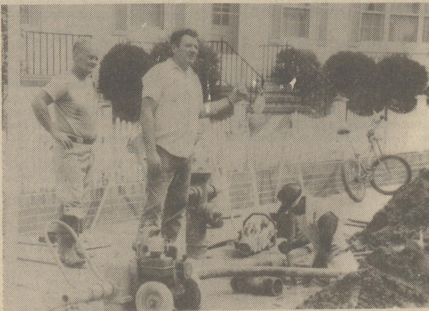
Jim Cooper, center, Street Superintendent for Harrington and his crew, Douglas Lahman, left and Ralph Benson, in the hole, worked on repair to the fire hydrant at the corner of Ward and Clark streets. Photo by HGF
