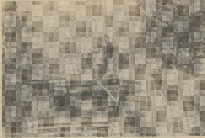
Delmarva Power workmen restore power to the homes in the area of Hanley Street in Harrington. Here, Durant Dennis, in bucket, trims limbs away from the primary lines in the alley between Hanley and Commerce streets. Photo by HGF
