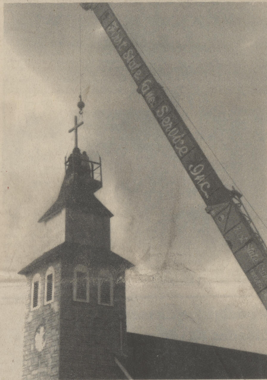
Grant & Son Roofing finds out "you have to go up to work for God" as they install new roofing to the St. Bernadette's Catholic Church in Harrington. Photo by David Dill.
