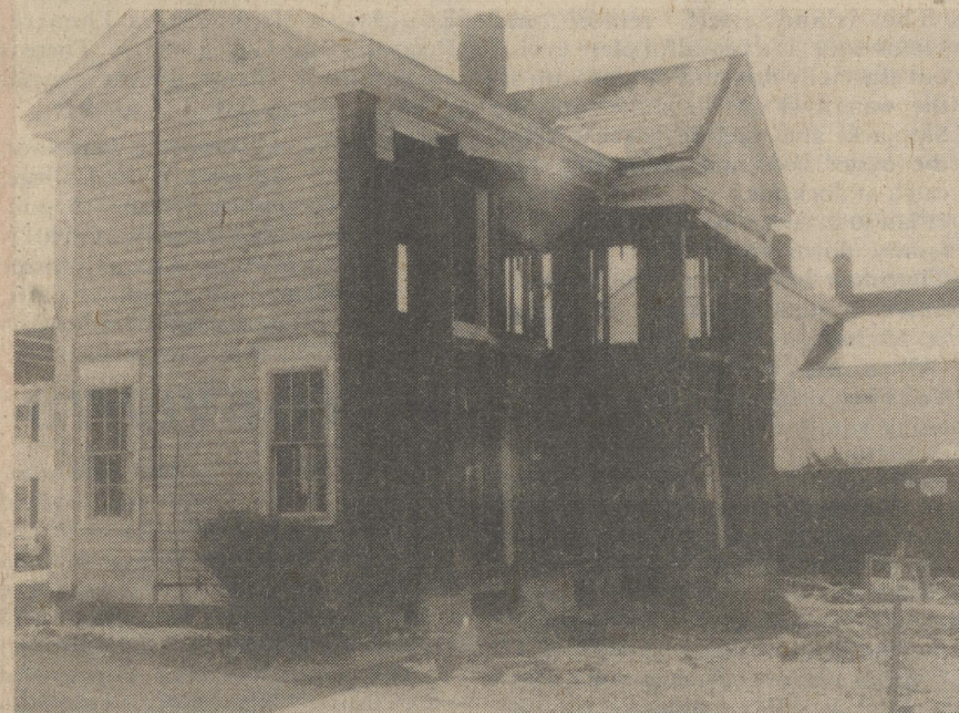
The house at the corner of Liberty and Fleming streets in Harrington belonging to Walter G. Lekites, III, has been partially taken down at request of City Council.
