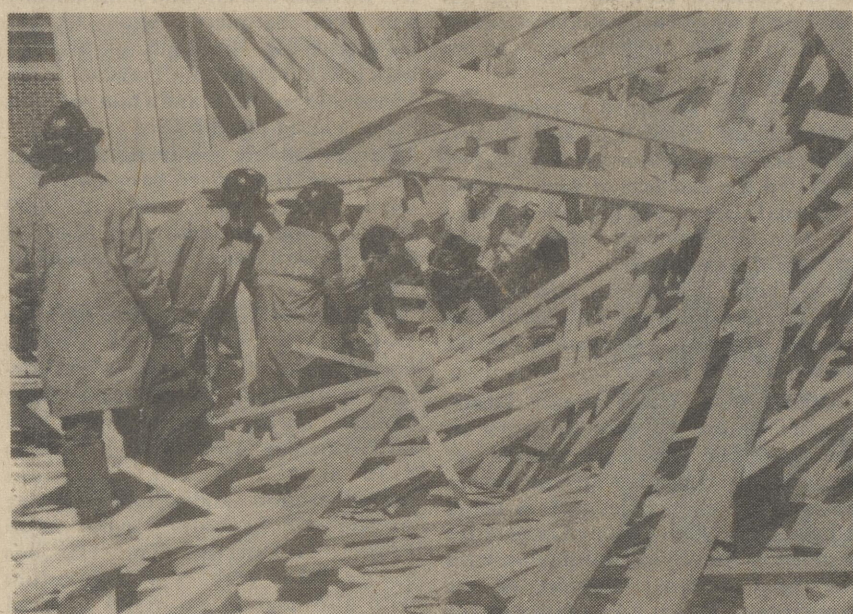
Harrington Firemen and Rescue Squad begin to free Randy Neelan of Lincoln, center of photo, following the collapse of trusses at the new addition on Calvary Wesleyan Church last Wednesday. "A gust of wind pushed the trusses down like falling dominos," said one observer. Neelan suffered a broken leg and some minor internal injuries. One other worker jumped to safety. Photo by HGF
