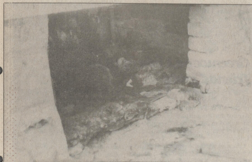
Underneath Maher's home is a composite of toilet tissue and sewage material that have flowed from a busted pipe. Photo by Bill Robertson
