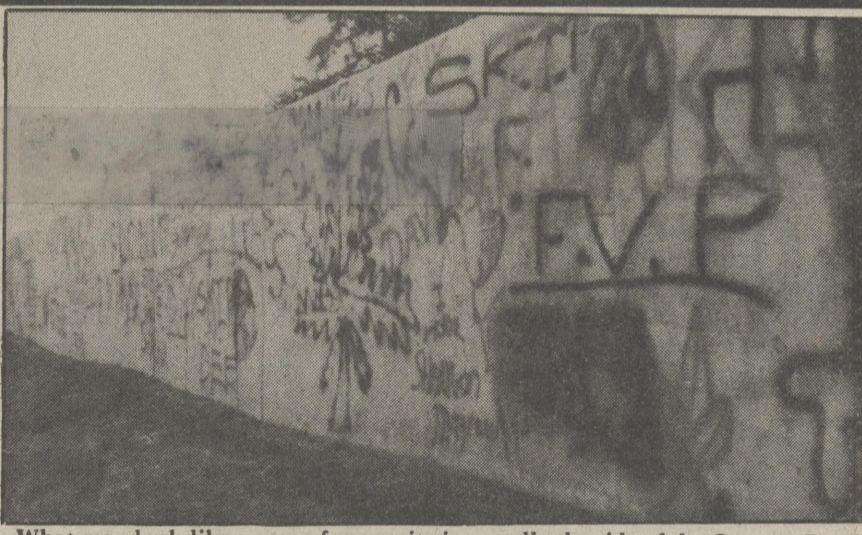
What may look like a scene from a city is actually the side of the Coursey Pond Bridge which has become covered by spray painted graffiti. Photo by HGF
