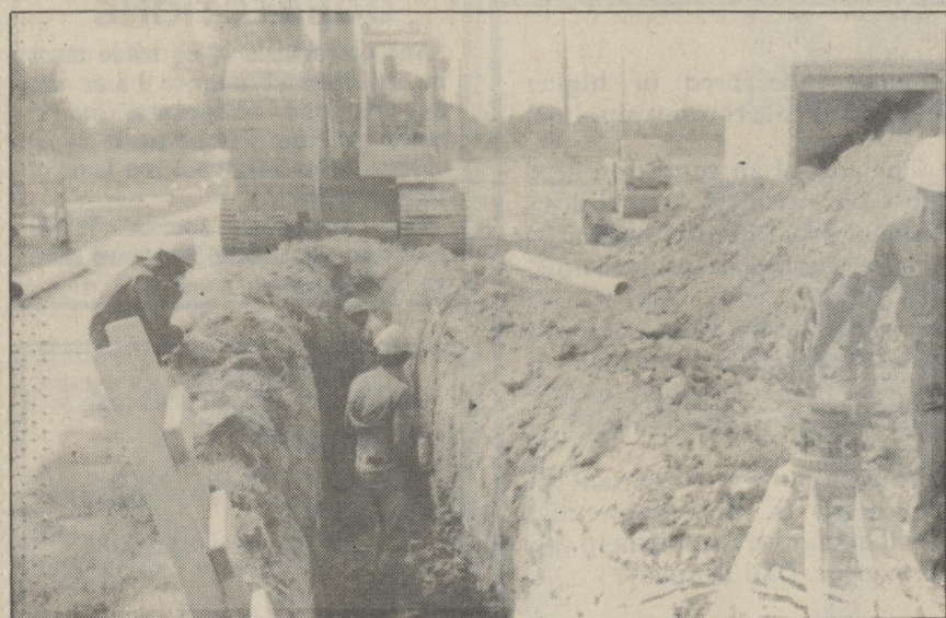
The West Mispillion and West Milby Streets are under construction with the addition of new water and sewer lines. This is a grant to the City of Harrington to enable these utilities to be available to the residents of that area. The cost is approximately $100,000. Photo by HGF
