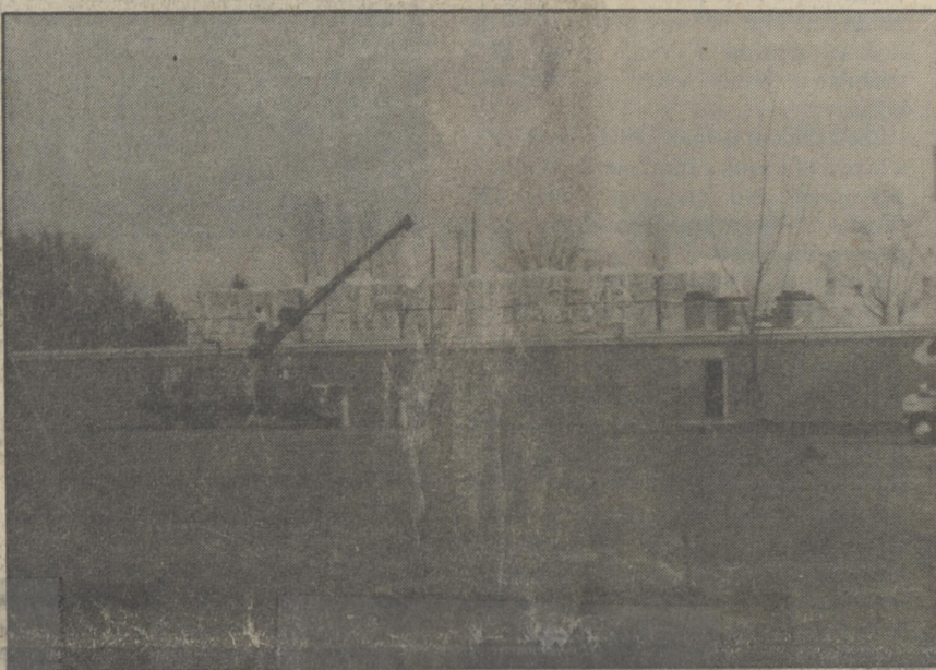
Due to the extreme disrepair of the roof at South B Elementary, work was begun last week to replace it. Photo by Don Mitchell
