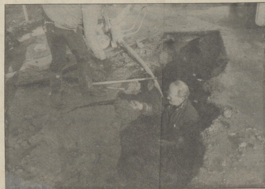
City employees were called out early Monday morning to repair a leak at the parking lot entrance to the Chipman School. Street foreman Jim Cooper hands Douglas Lahman a gasket for the pipe where the leak occurred. Photo by HGF.
